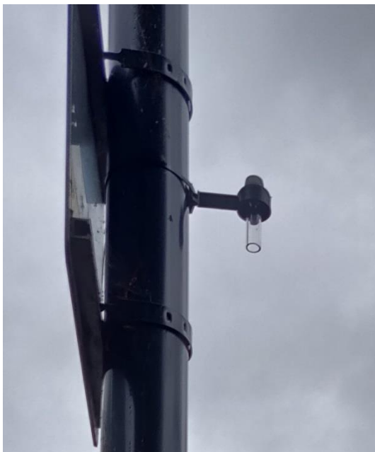
A diffusion tube installed using a spacer and placed in freely-circulating air
