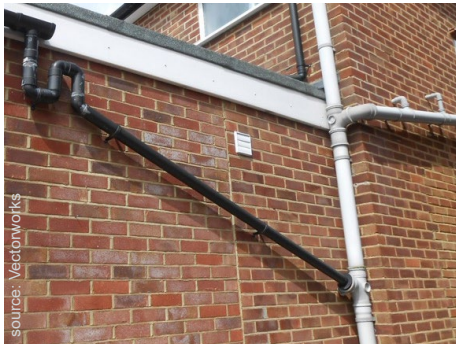
Drain pipes not designed in from the start are likely to detract from the facade ❌
