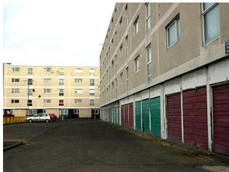
Undercroft parking eliminates active frontage on the ground floor ❌
