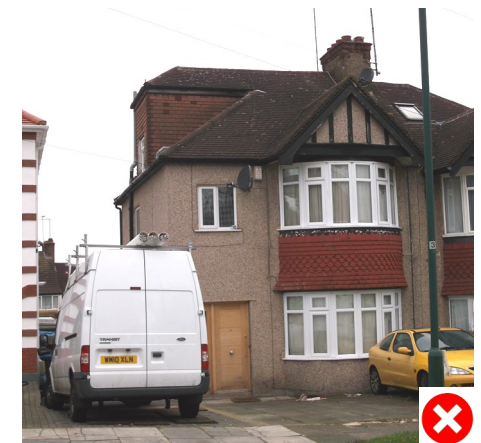
Side dormer that distorts the character of the roof and the building
