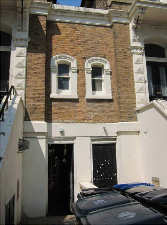
Typical link block between main buildings, with ground level access gates to rear gardens
