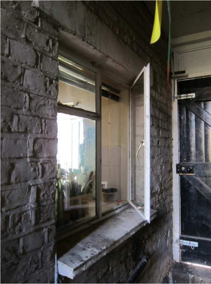
Ground floor side elevation steel kitchen window, with gate to street on right (15 Princess Road)
