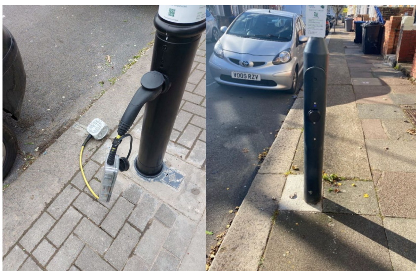
Examples of the EVCPs Installed within Bollards and Lampposts around the Borough (Source: LBB)
