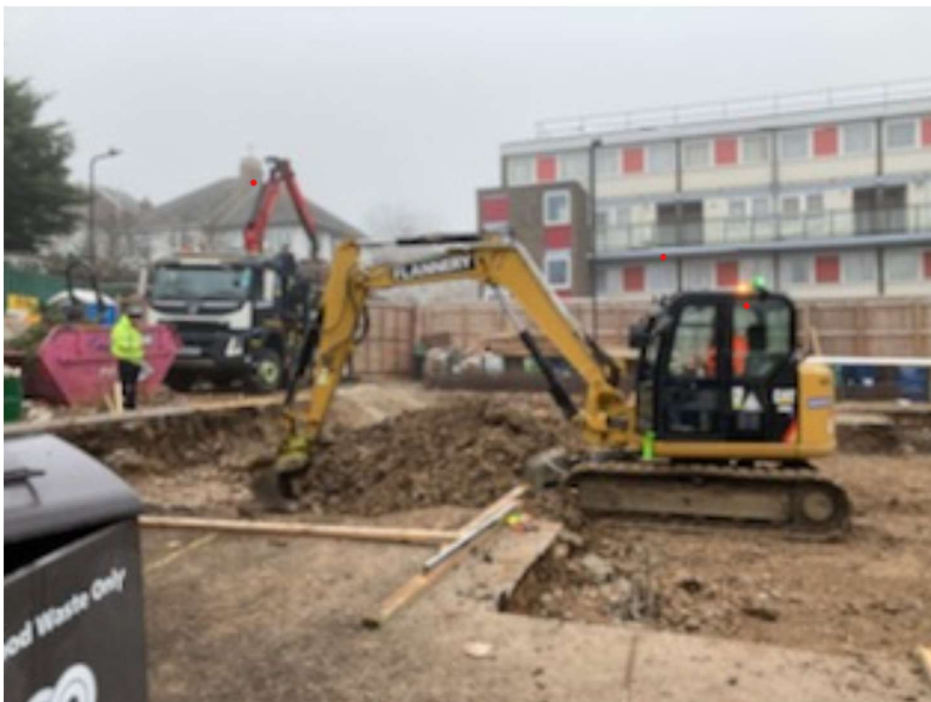
Image showing work underway at Hindhurst Court, December 2020. Planned end date: June 2022 (Source: LBB)
