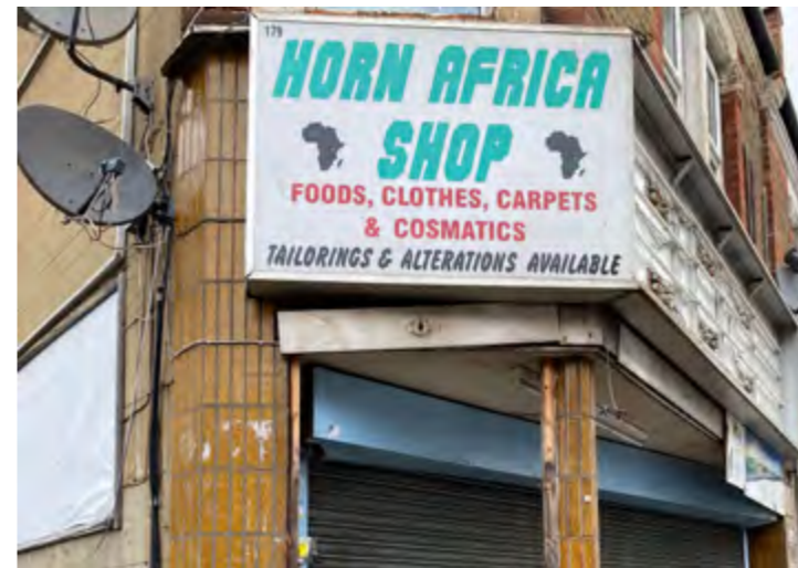
Church Road - defunct illuminated box sign
